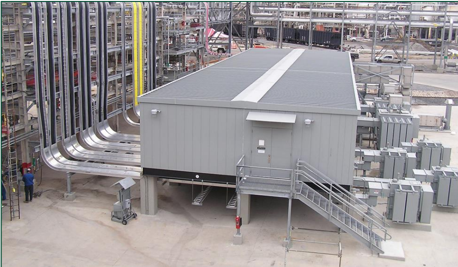
Power Control Room
