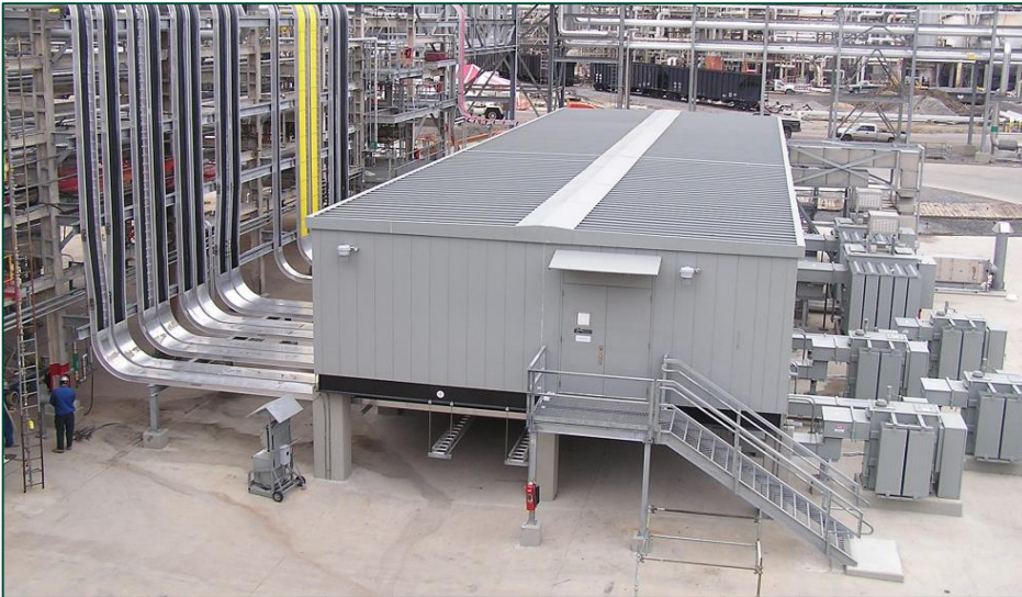
Power Control Room
