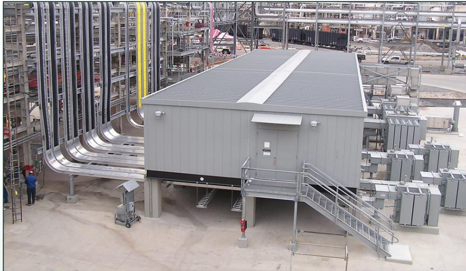
Power Control Room
